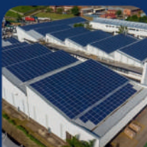
Industrial Solar Rooftops
