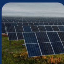
Ground Mounted Solar Systems
