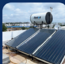
Solar Water Heaters
