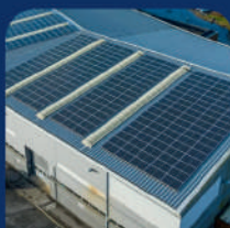
Commercial Solar Rooftops
